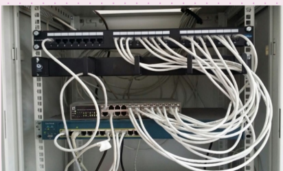
Patch panel in stikala (vir: lasten)
